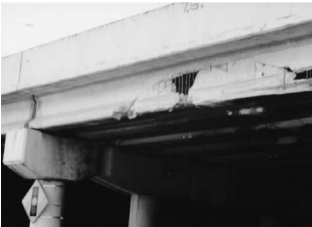
Figure 3.1. Examples of damages: corrosion (top) and vehicle collision (bottom).
